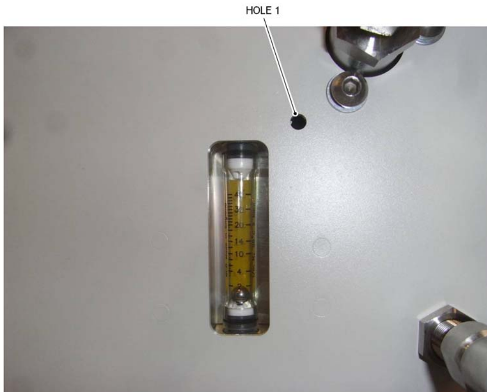
Figure 16 - Nitrogen flow meter
